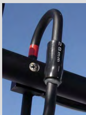
Sealed feed point
